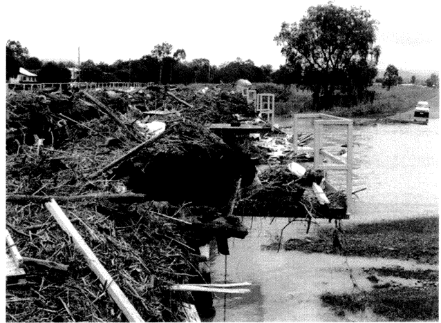
The Grantham Rail Bridge that separated the lower flood affected section of the Township from the higher relatively flood free areas.
